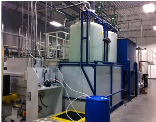
Shown: CRS-F-15-6FP-AX-4-N4-DC-FL-DL 15 gallon per minute fluoride removal system with equalization tank (not shown) and a 460 VAC PLC based indoor rated system.
